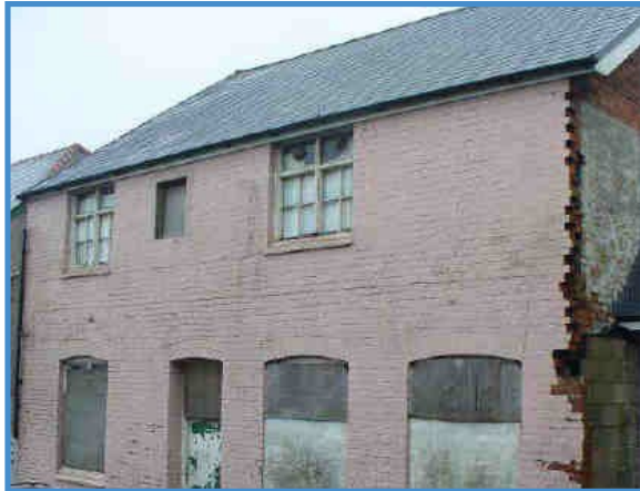
Vacant buildings on Williams Terrace
